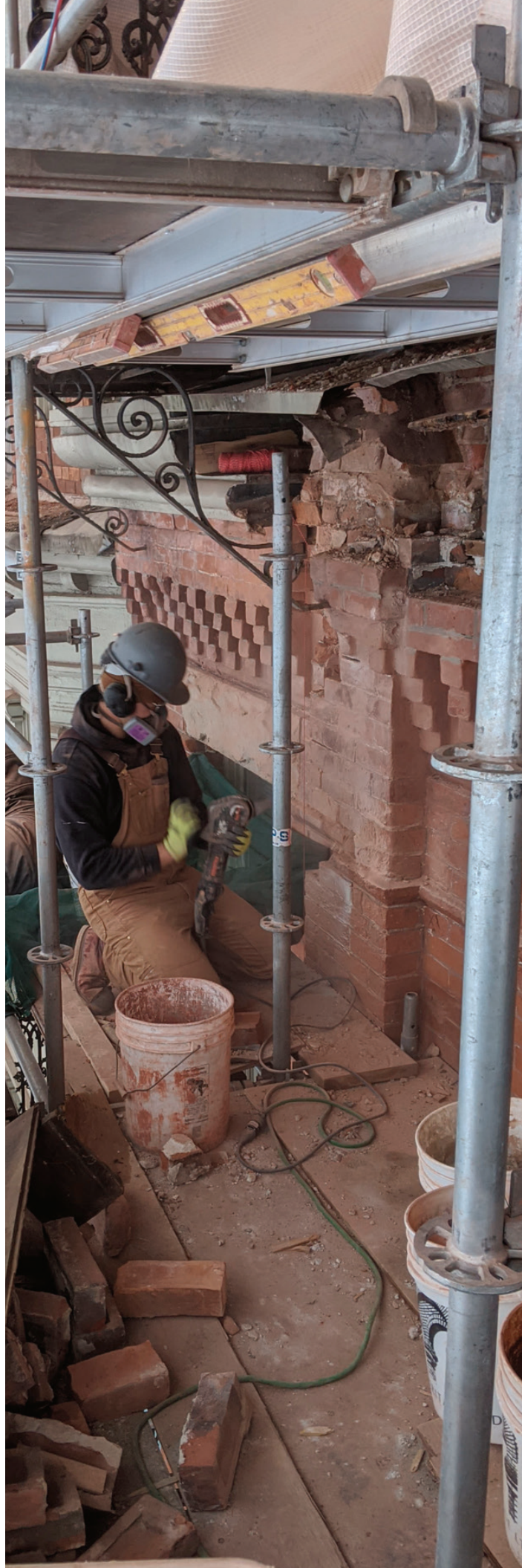
Jeremy Pfuetzner, James Strachan Award for Craft nominee, hard at work repairing damaged corbelling and brickwork.
