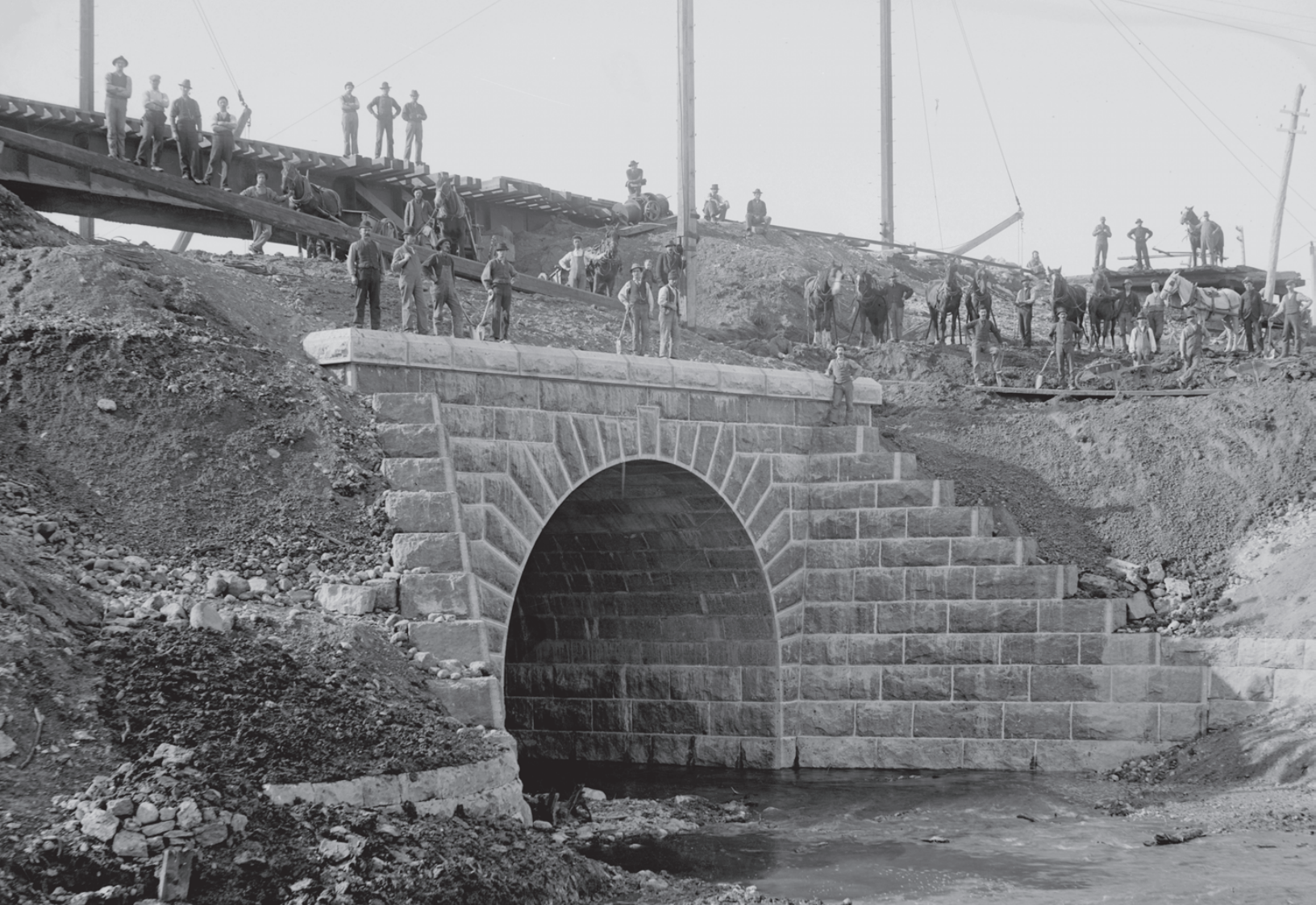
▲ Construction south of Newcastle. Photo W. H. Chaplin, 1906, Courtesy Newcastle Village and District Historical Society
