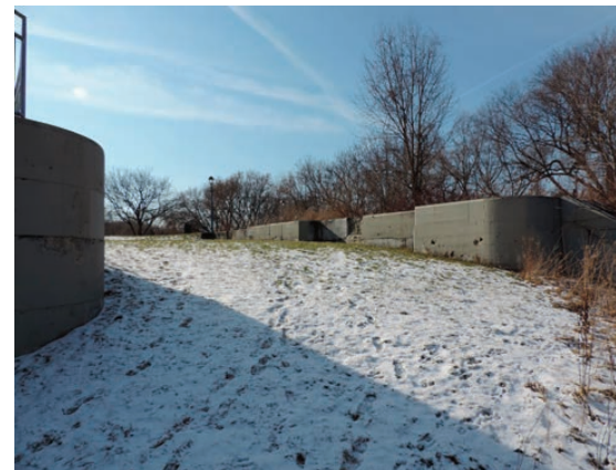
▲ Remnants of the Newmarket Lock. Costing almost $1 million, there was never enough water for navigation on the canal. Photo Gordon Prentice, 2018
